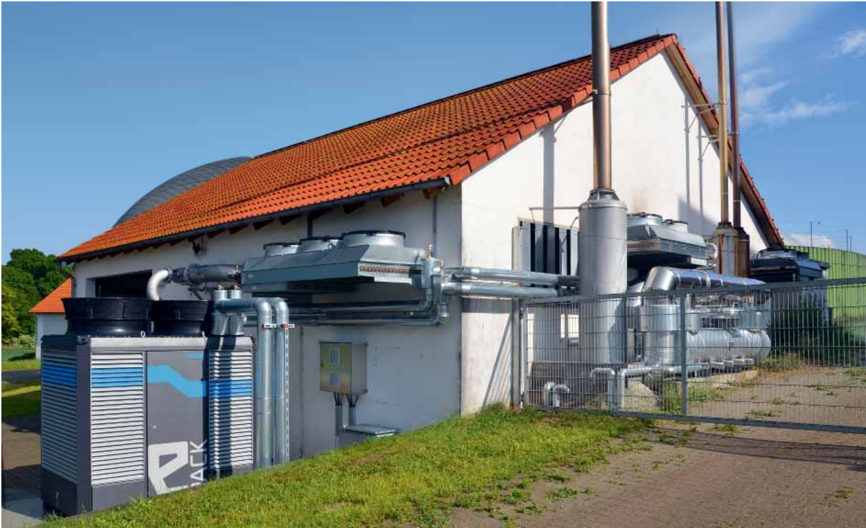
Use of Orcan Energy's compact ORC module in an anaerobic digestion plant.
